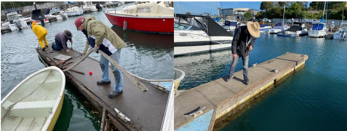
Pictured: Derrick Kershaw, Hardy Weller, and Colin Diggins commencing removal of rotted material.
